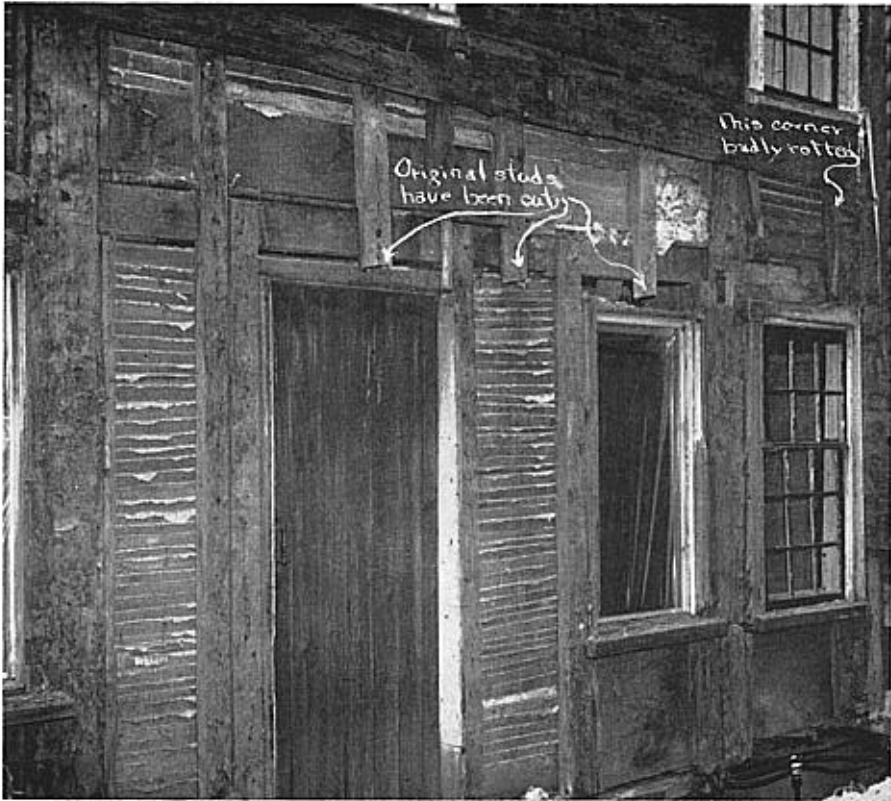
FIG. 3. EXTERIOR WALL SHOWING POSTS AND STUDS (OR SIDE BEARERS) CUT OFF BELOW GIRTS, SEVENTEENTH-CENTURY CONSTRUCTION
