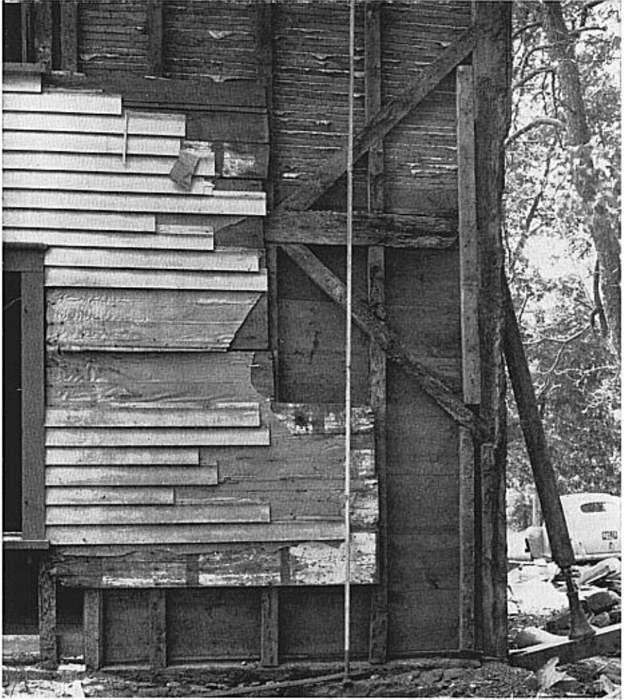
FIG. 4. EXTERIOR WALL SHOWING CORNER POST, GIRT, STUDS AND BRACES, AND SILL, EIGHTEENTH-CENTURY CONSTRUCTION
